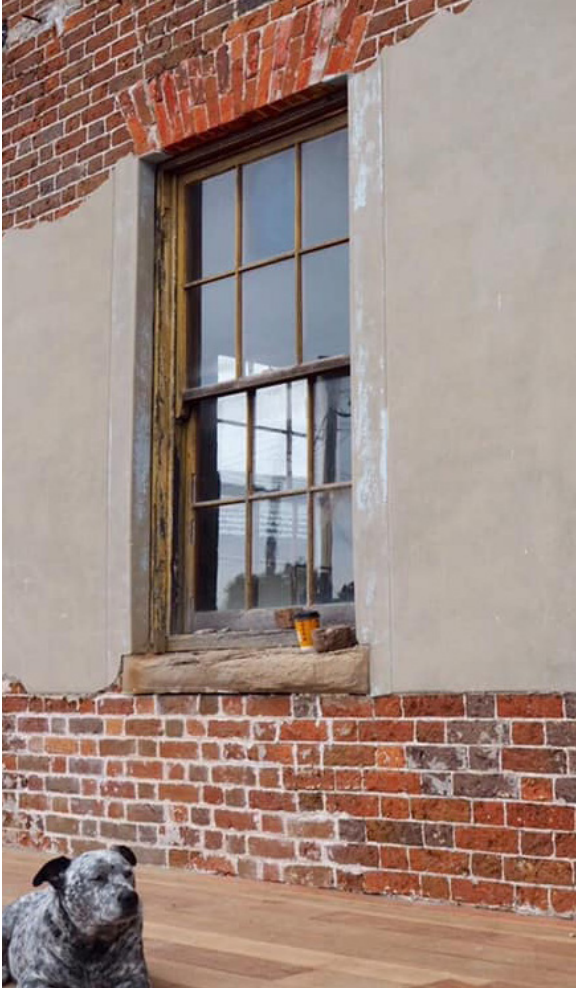
Render being removed from original convict bricks at Keeravale, West Wollongong Image: David McReady (Facebook)
