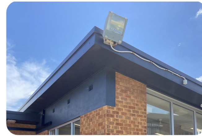
New FC fascias and soffits to eaves of hall building roof. Finish of FC fascia and soffit to match colour of roof capping
