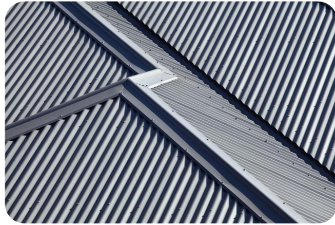
RF-01: Colourbond Ultra roofing to new additions. Colour in Shale Grey. Profiles of new gutters and downpipes to match existing profiles. Finish of gutters and downpipes to match fascia
