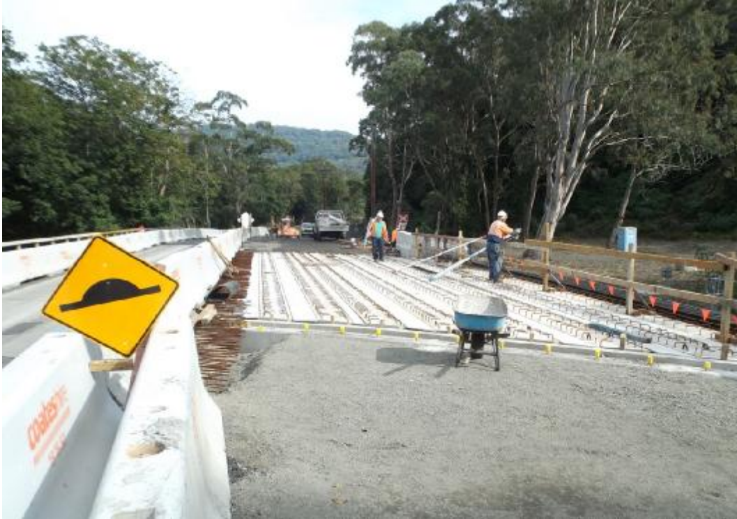
Image: Work progressing on the replacement of William James Bridge, Mt Kembla
