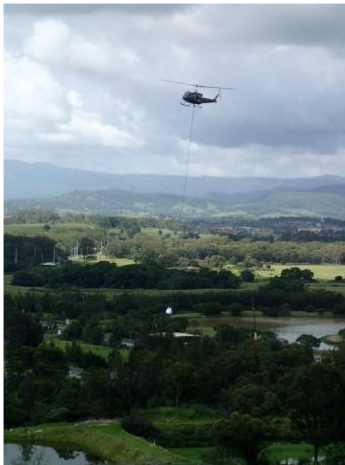
Image: A helicopter used as part of the finalisation of the new landfill cell at Whytes Gully
